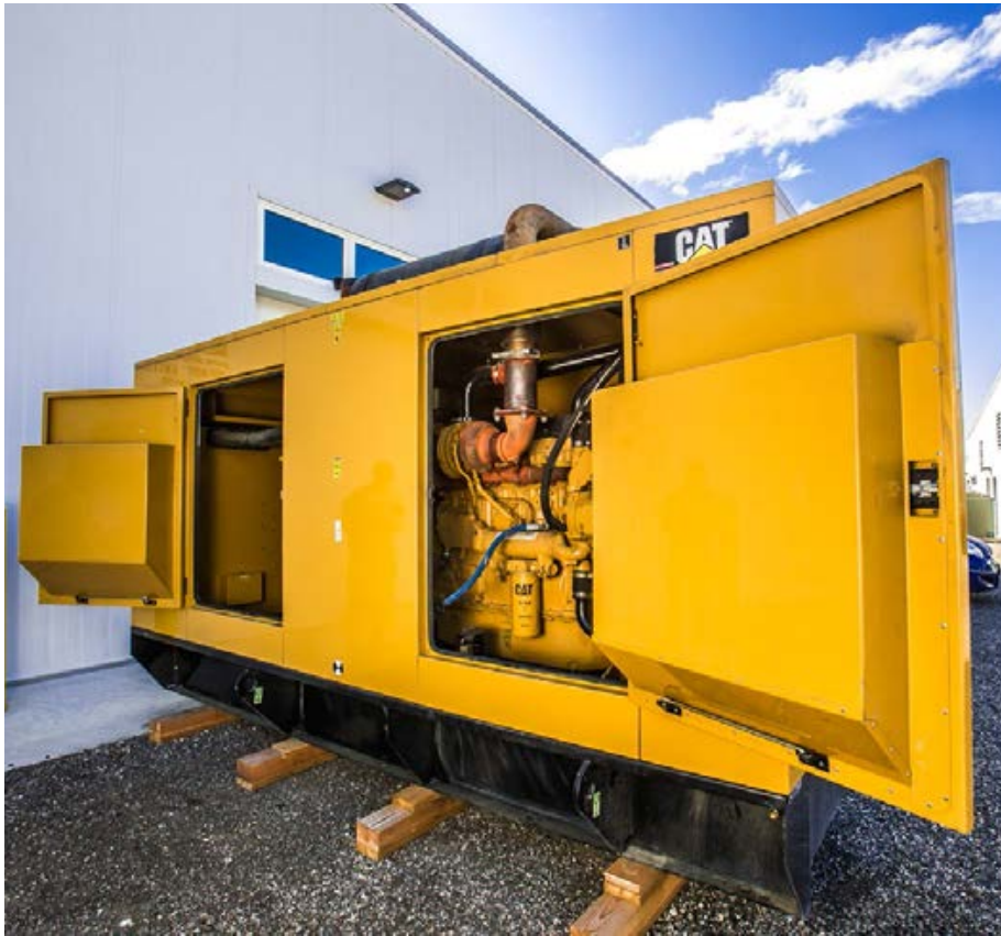
Figure 10: The C15 Caterpillar diesel generator.
